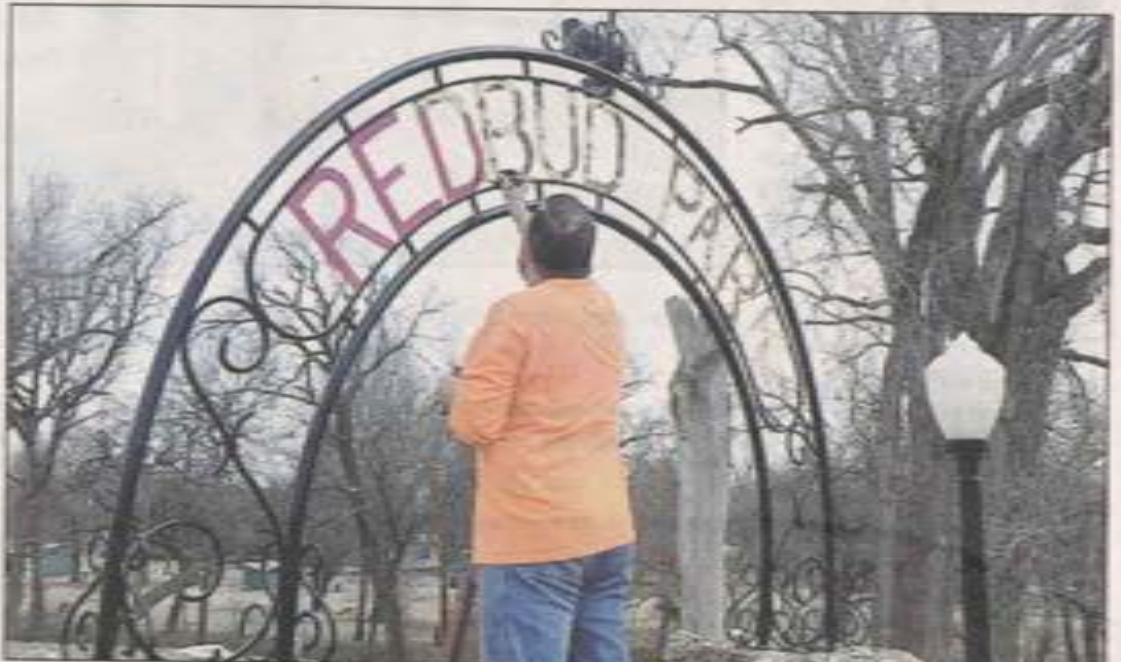
FRESH PAINT JOB: Marlow street department supervisor Jerome McGavin gives the entrance sign at Redbud Chapel a fresh coat of paint in February when the department was able to take advantage of warmer weather.
